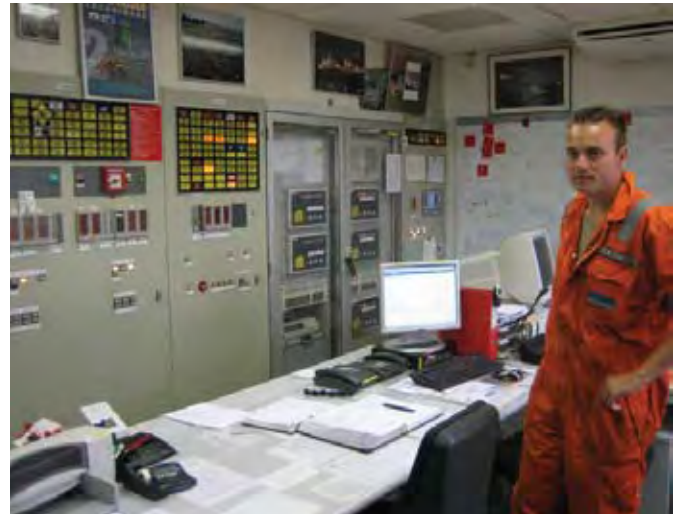
Waalwijk control room – as at 1 June 2009 24,266 LTI free hours under the operatorship of NPN.
